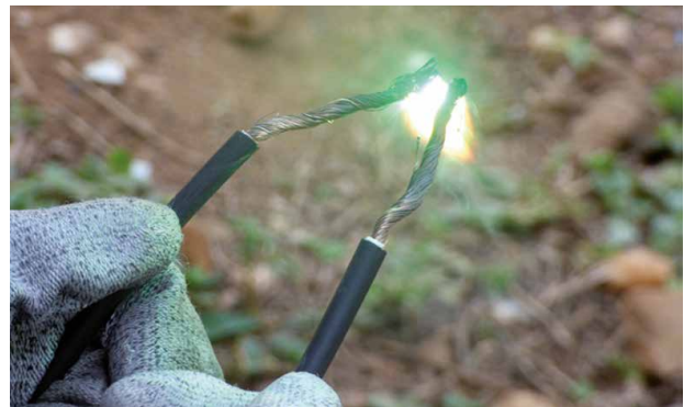
Figure 14: Example of an electric arc at the terminals of a 200 WP module under 1000 w/m 2 sunlight -
