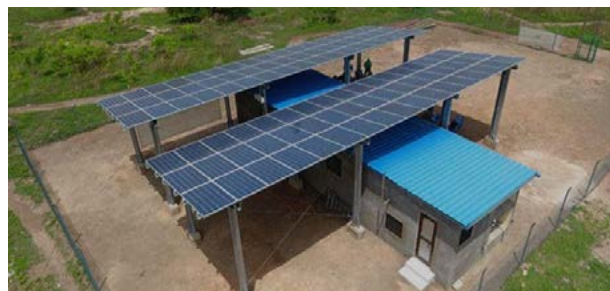
Figure 2: A 54kW microgrid facility in Kudorkope, Ghana. Source: Volta River Authority, Ghana.
